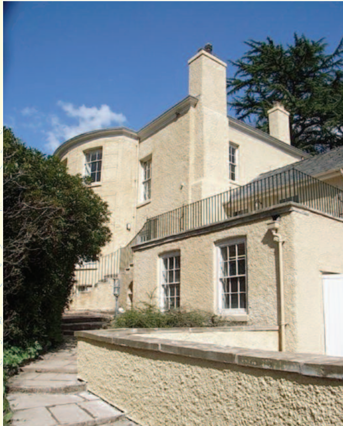
Restoration of Samuel Gregg's House at Quarry Bank Mill for the National Trust
